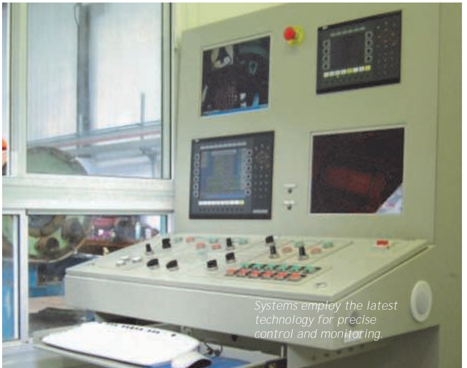
Operators have all controls to hand, and are able to see directly into the jacking shaft.
